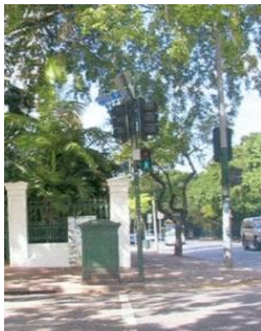
Figure 39 - City Electric & Light (CEL) Company Junction Box (outside 19 George Street) (Urbis 2017)
