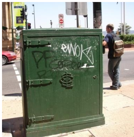
Figure 40 - City Electric & Light (CEL) Company Junction Box (outside 33 Queen Street) (Urbis 2017)
