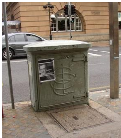
Figure 41 - City Electric & Light (CEL) Company Junction Box (outside 125 George Street) (Urbis 2017)
