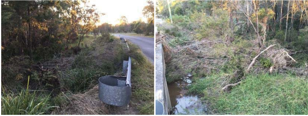
Figure 15: Pineview Road culvert upstream debris following 1 May 2015
