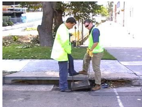
Plate 9 Lift grate above the support frame
