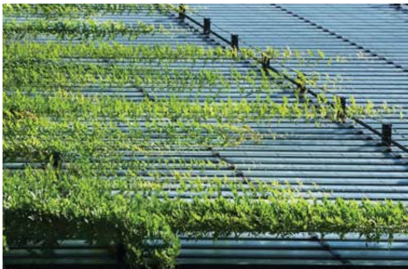
wire trellis catenary
