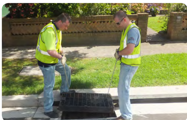
Photo 9 Lift grate above the support frame
