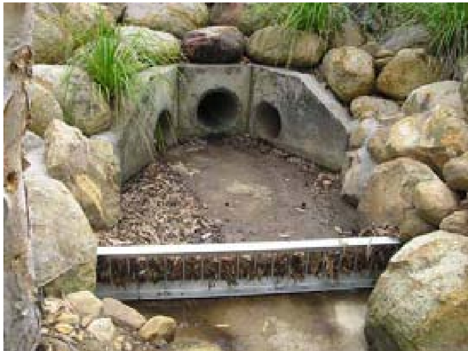
Figure 3-6 Example of a Trash Rack
