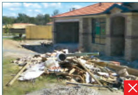
Poor litter and building waste storage
