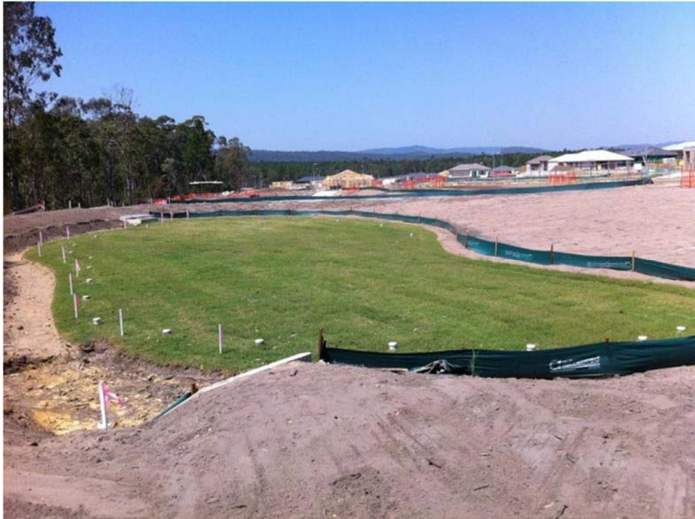
Photo: Bioretention B1a in Precinct 1 with protective turf in place
