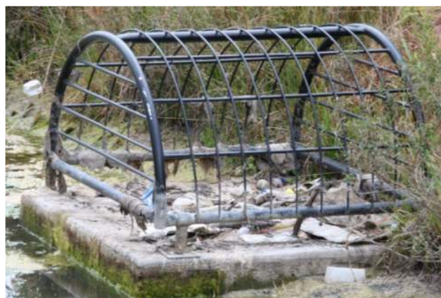
Figure 16 Litter blocking outlet pits
