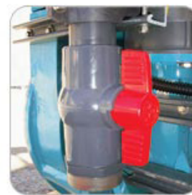
Inlet & Discharge Plumbing With Pipe Support
