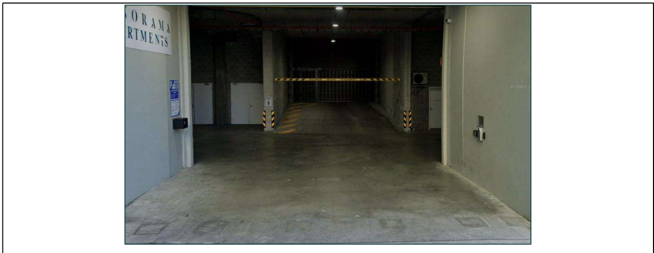
Figure 1 Existing Wall Mounted Intercom System
