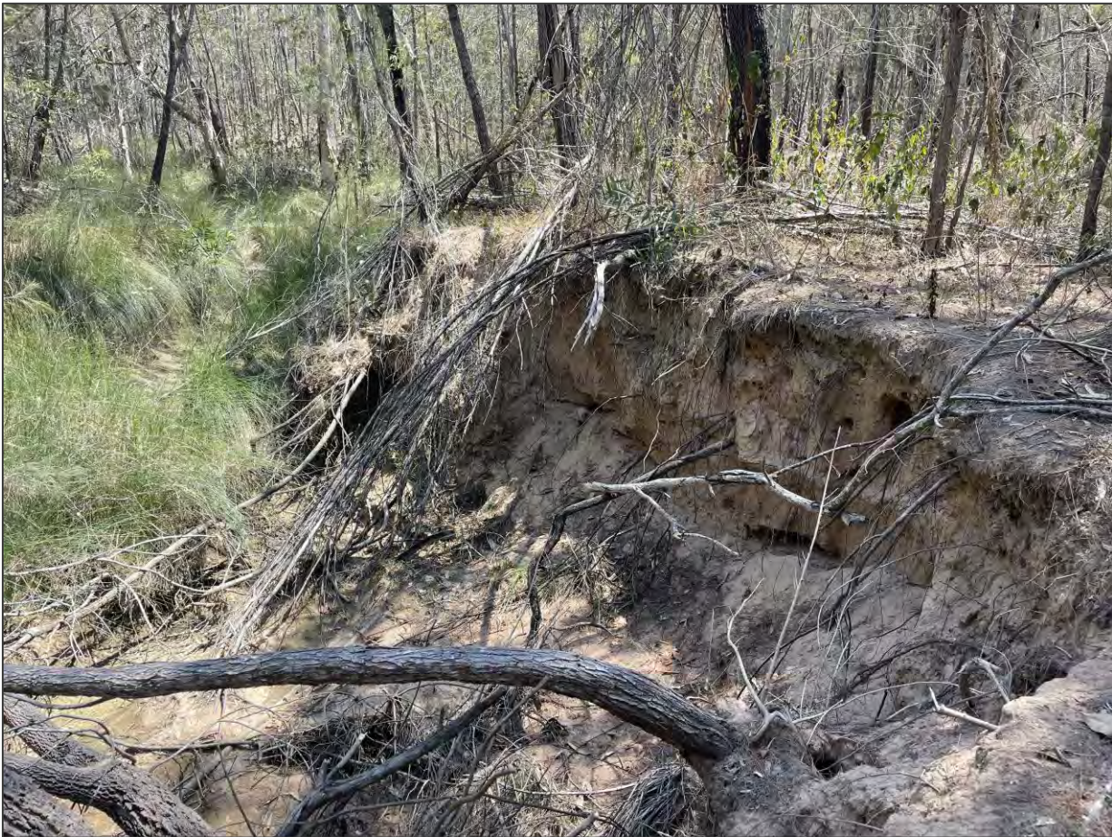
Figure 4.1: Existing Eroded Creek Line within the Site
