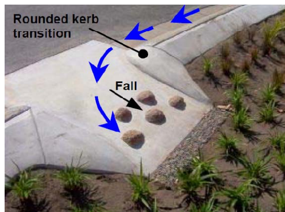
Photo 20 - Bioretention Garden Inlet
