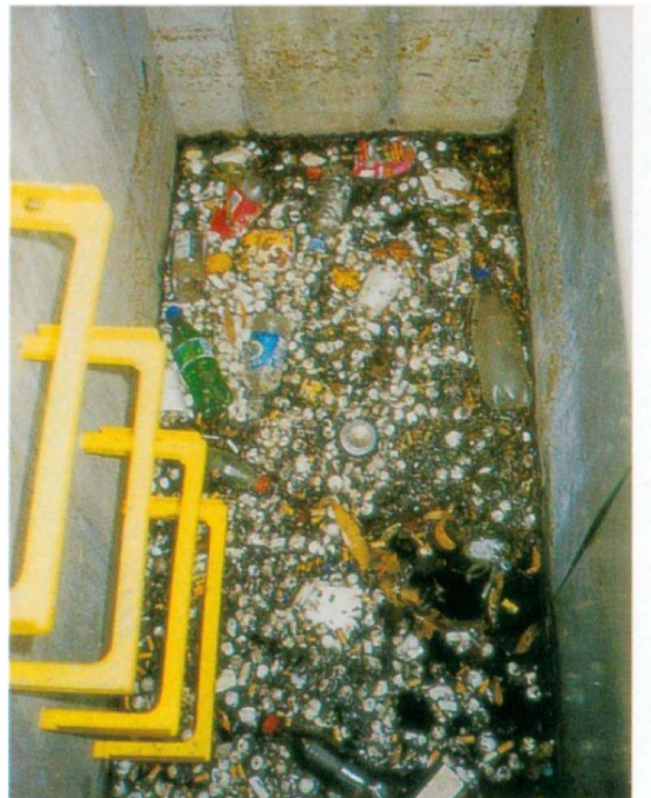
Photo 15 - Inside a Humeguard showing trapped Pollutants
