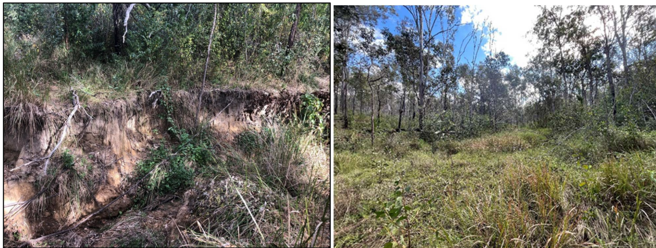
Photo set 15: Eroded drainage feature (drainage line 8) (left) and overland flow path (drainage line 8) (right).
