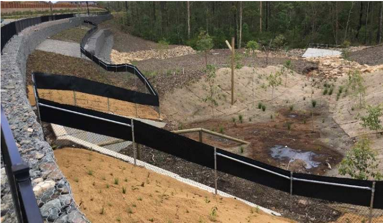
Image: Fauna exclusion fence to direct fauna towards culvert entrances
