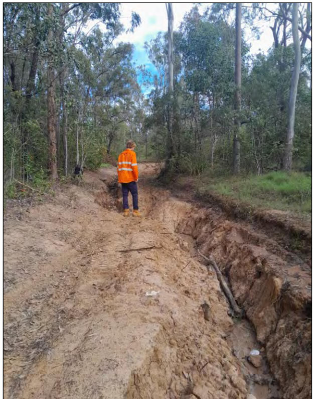
Photograph 4: Unsealed track to Bores 1 and 2 displaying signs of significant erosion.
