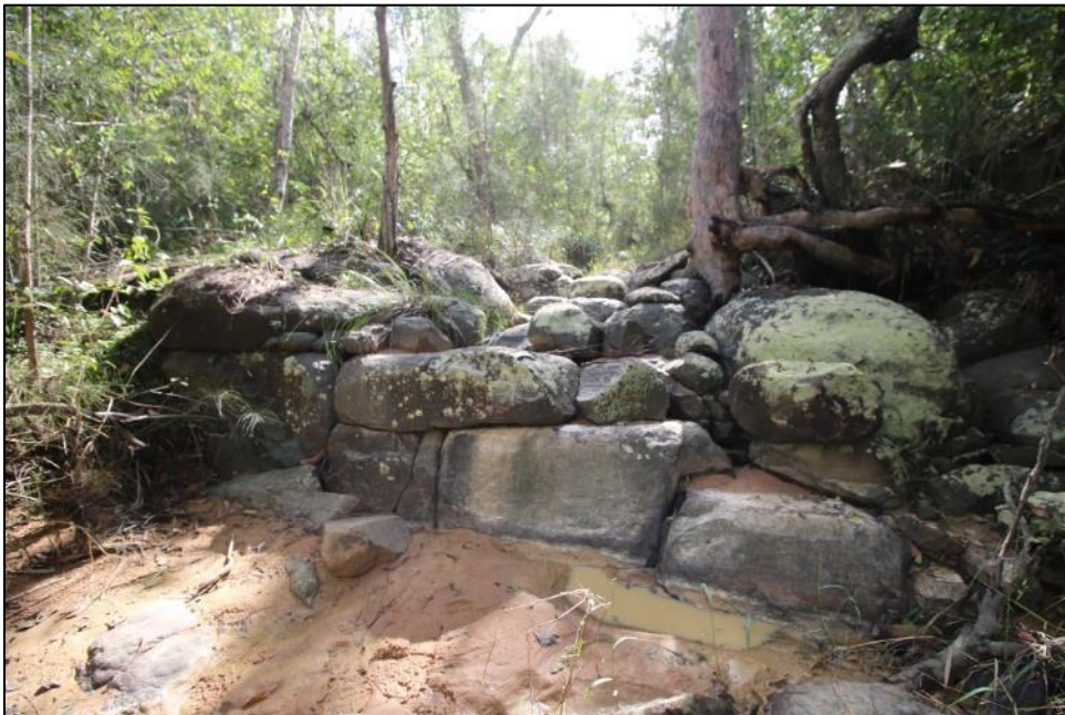
Site C3. Large rock barrier (single 0.9m vertical drop and 1.6m drop overall) that is a significant barrier to fish in the middle of the dry mapped waterway (other than the occasional very small puddle from recent rain).
