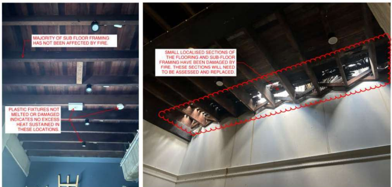
Figures 8 & 9 – Upper -Level Sub-Floor Timber Framing, Figure 9 Shows Small Localised Damage to Joists, Nogging and Flooring.
