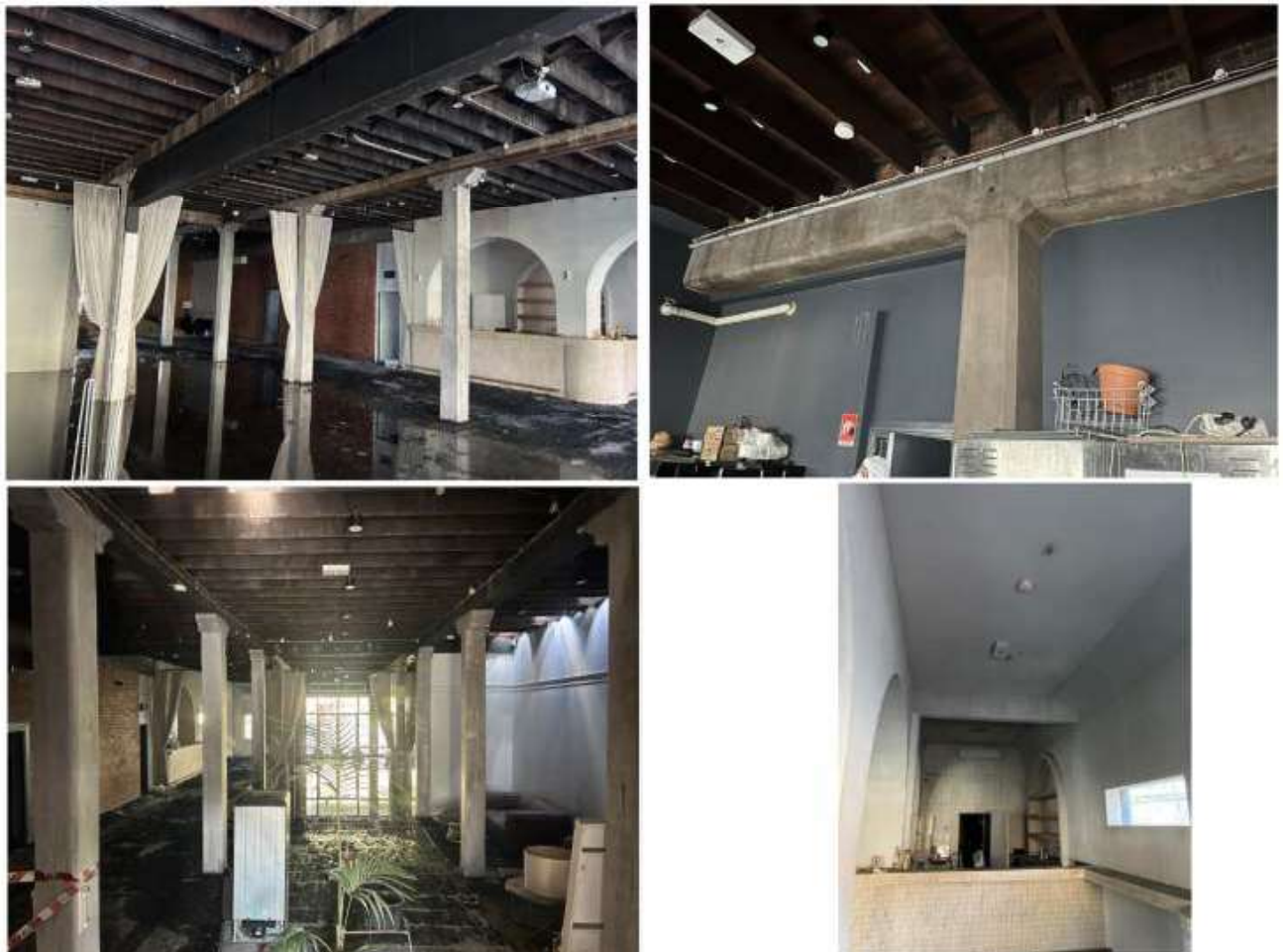
Figures 10, 11, 12 & 13 – Lower-Level Structural Elements, Mostly Undamaged/Unaffected by Fire.
