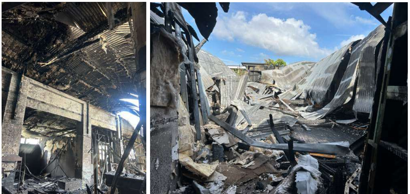
Figure 3 – Photos Taken Post Fire Event, Showing Full Roof Collapse and Extents of Damage.
