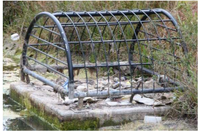
Figure 16 Litter blocking outlet pits
