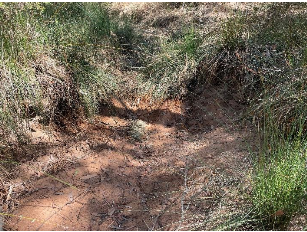
Location 15 – Bank Erosion and Split Waterway
