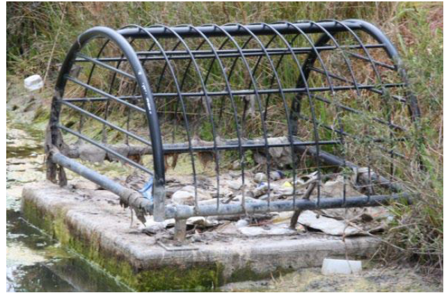
Figure 16 Litter blocking outlet pits
