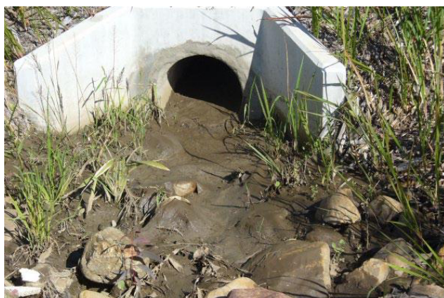
Figure 17 Sediment accumulated at an inlet
