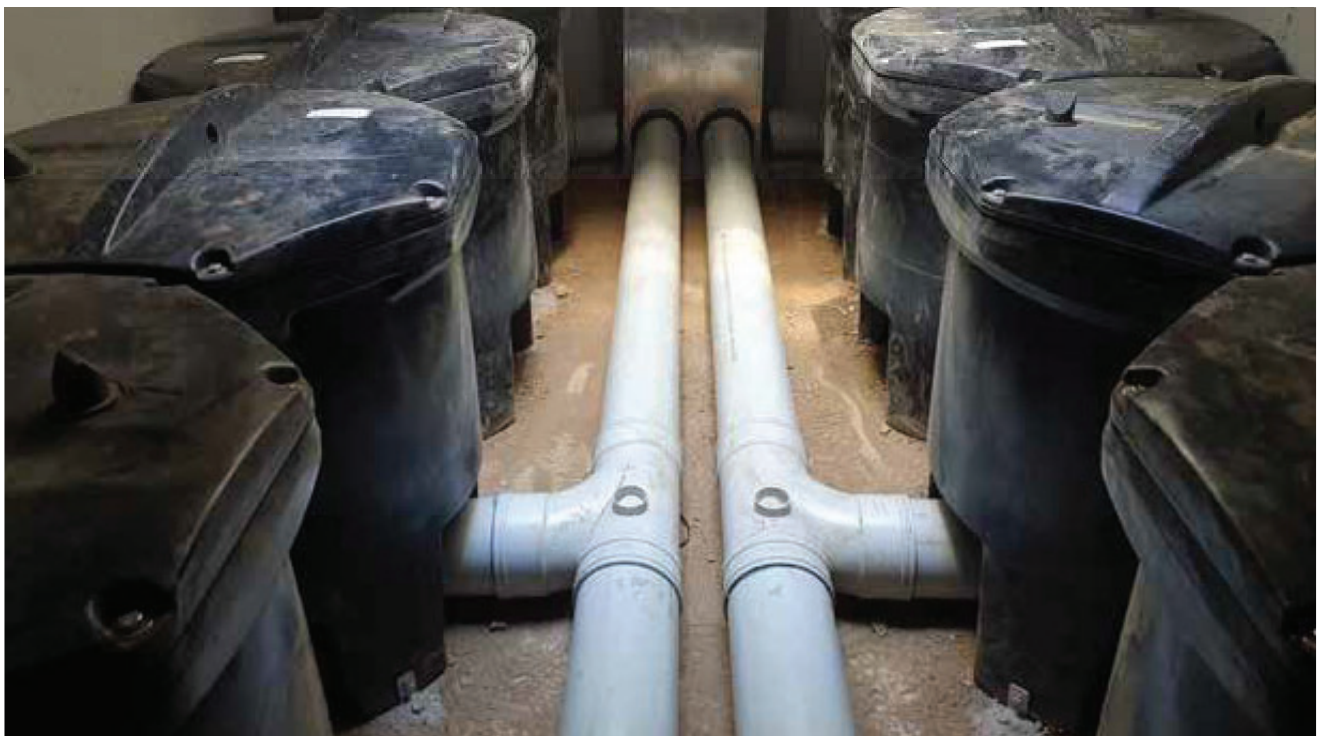
Figure 1 - SPELFilters in a concrete chamber / vault
