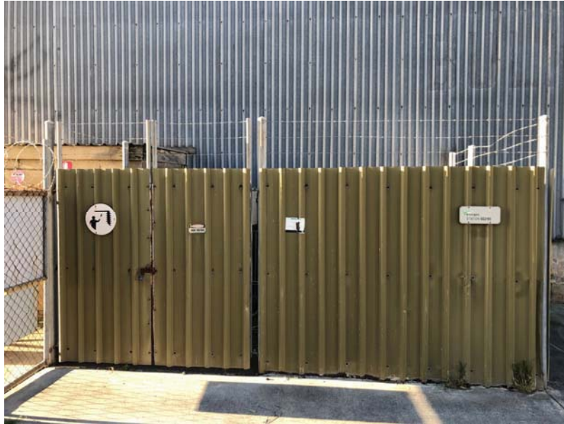
Photograph 19: View of historical transformer located at the front of N shed
