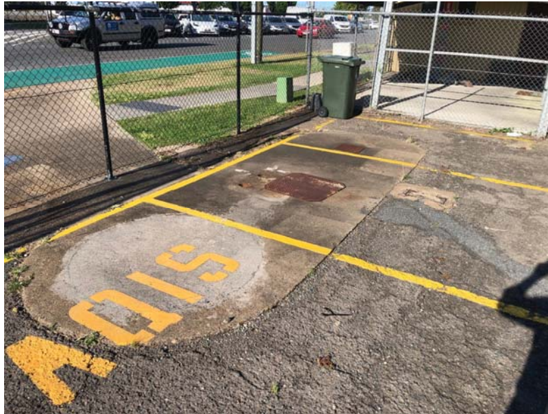
Photograph 17: View of possible former underground fuel storage tank in the northwest corner of the site
