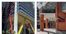
High quality finish to the surface of columns, with column form, material and colour forming part of the overall building facade
