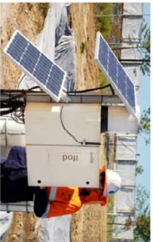
IFOD Flow Dosing Unit (custom built)
