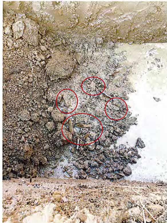
Plate 2: Observed ACM Fragments Post-Excavation
