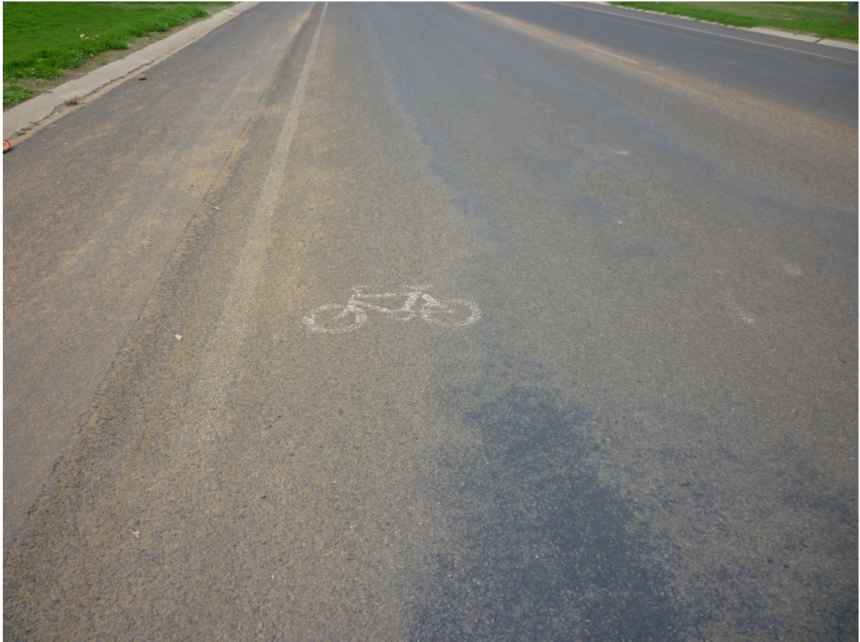
Figure 2.7: Cycle Lane Markings Worn-Away
