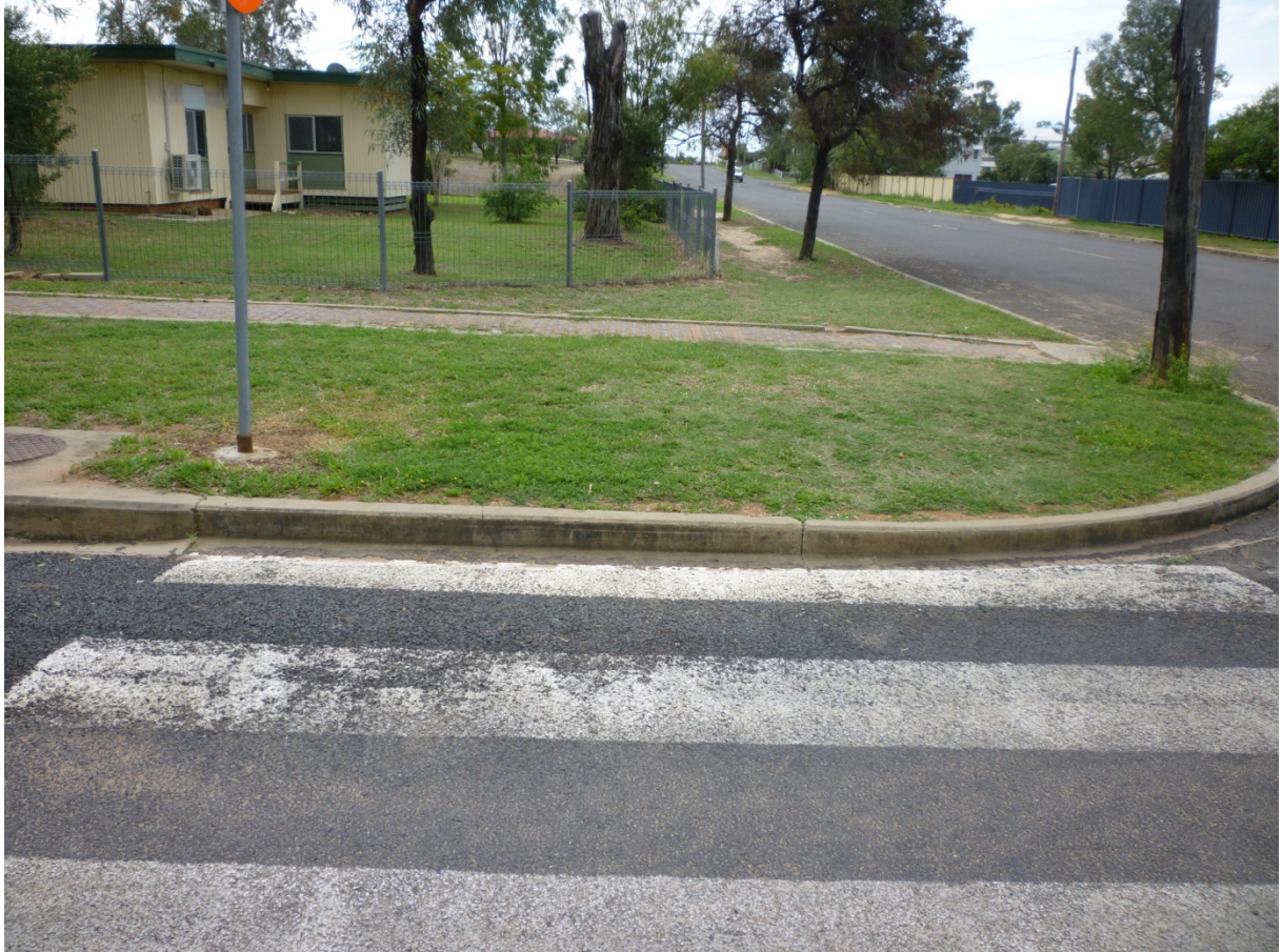
Figure 2.5: No Connection between Pedestrian Crossing and Footpath
