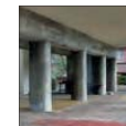
Columns that are undressed and have poor finishes that are inconsistent with the design and quality of the building facade
