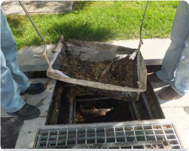
Photo 14 Lift the bag from the stormwater pit
