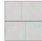
Building materials that lack expression or creative use, and do not contribute to the building's identity
