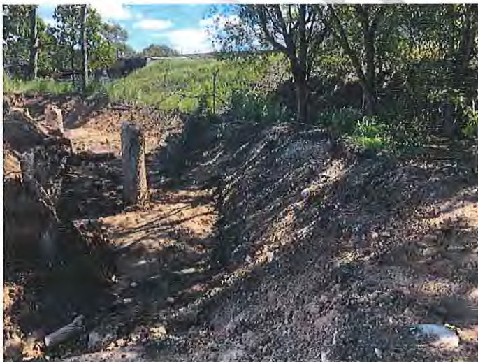
Photograph 3: A view of the northern vegetated portion of the site facing towards the west, with the bund material that contains C&D Waste and ACM pictured in the right of the photograph. (Image Date: 3 July 2019)
