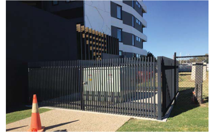
03 - Existing padmount on Lot 302
