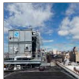
Unconcealed building services and mechanical equipment visible on tower rooftops
