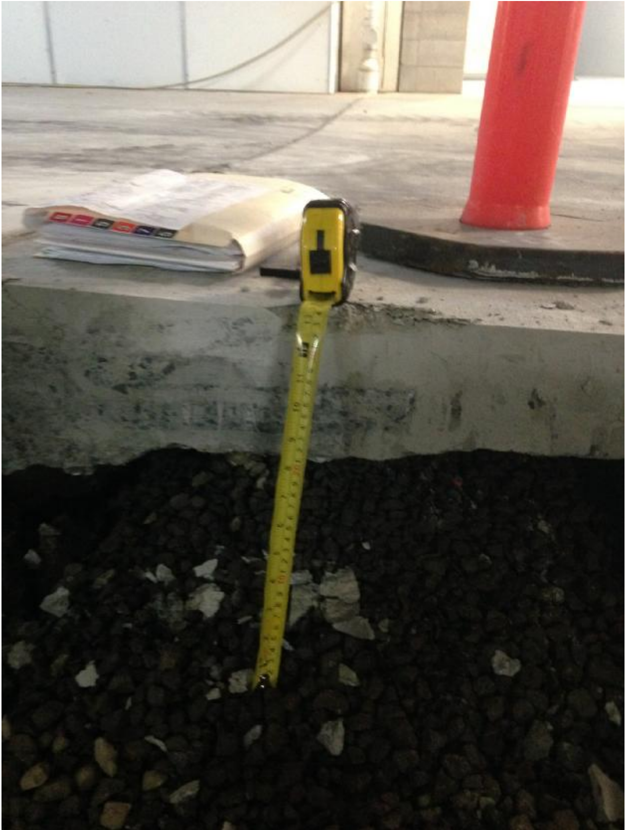
Photo 1 – Void under slab
