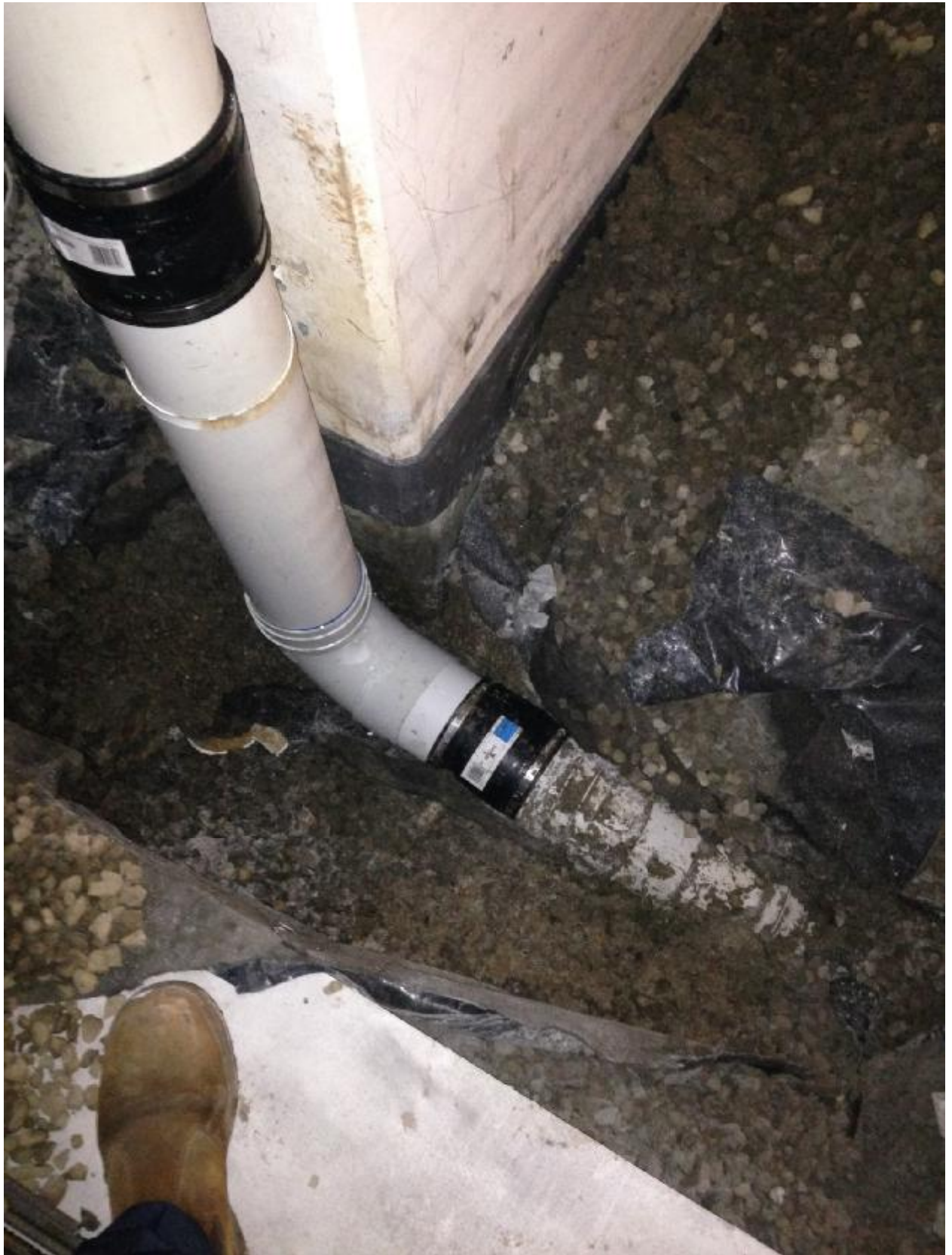
Photo 13 – Repair undertaken to broken roofwater pipe
