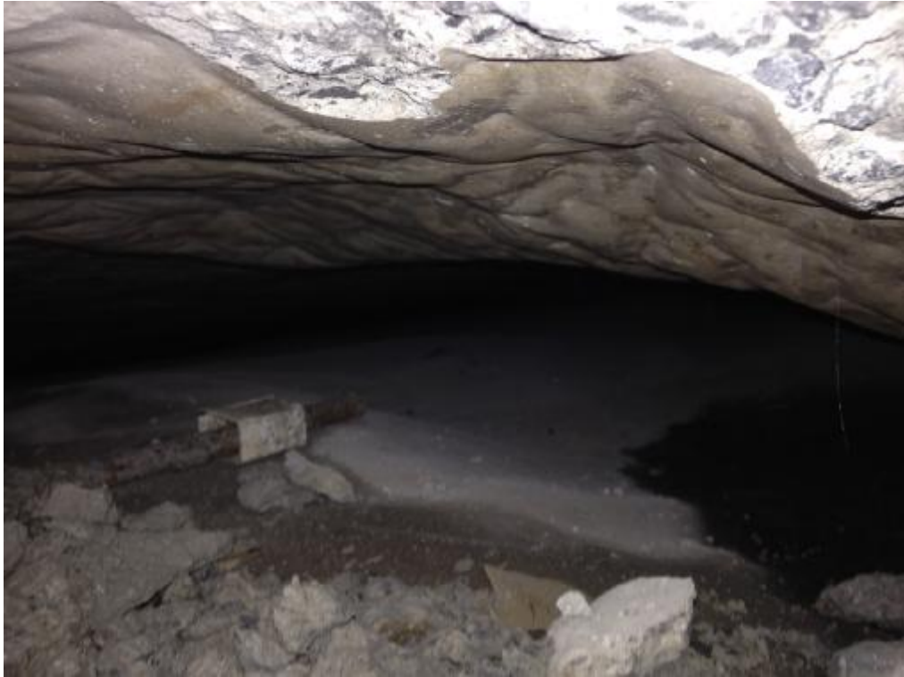
Photo 10 – Void under slab
