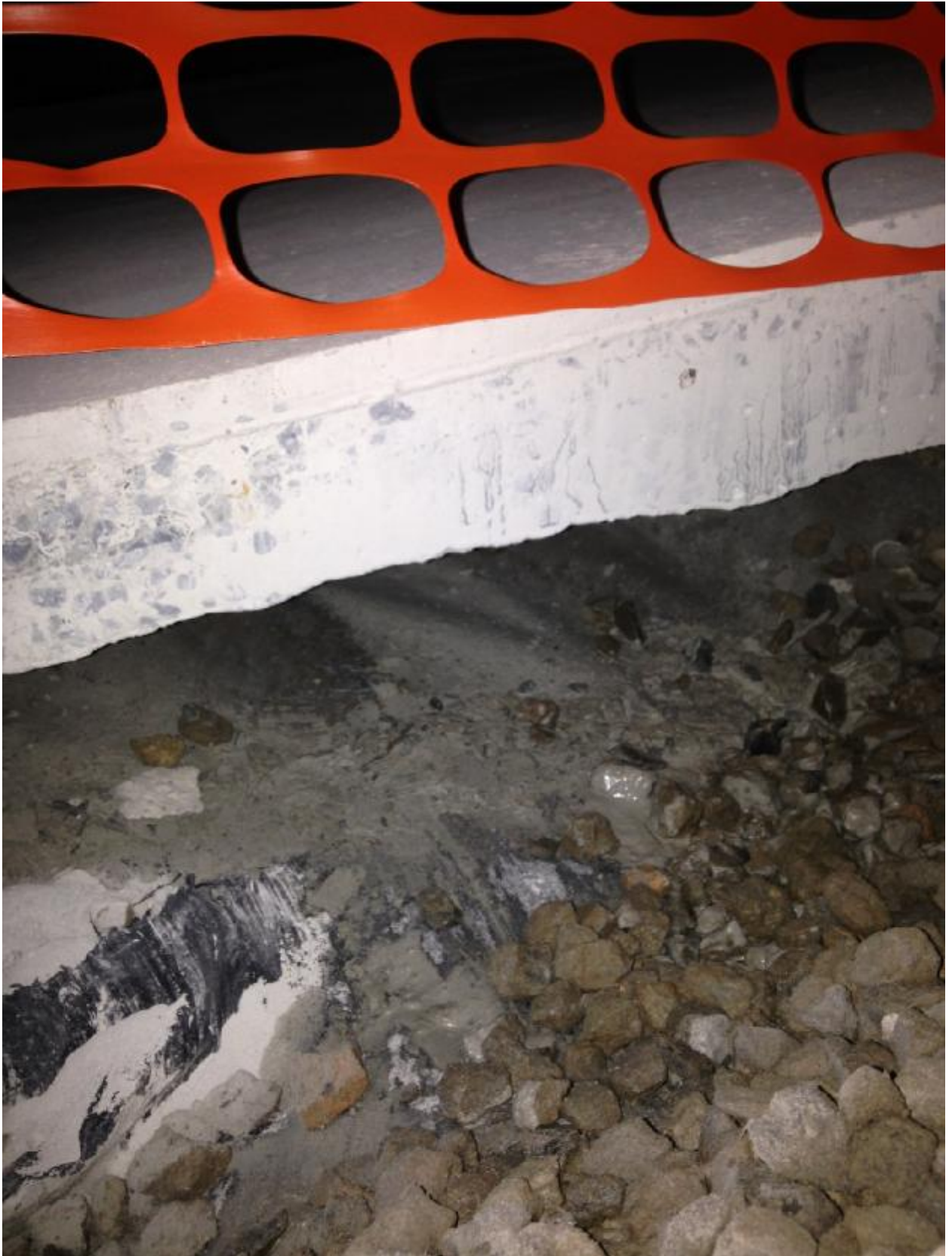
Photo 14 – Void under slab
