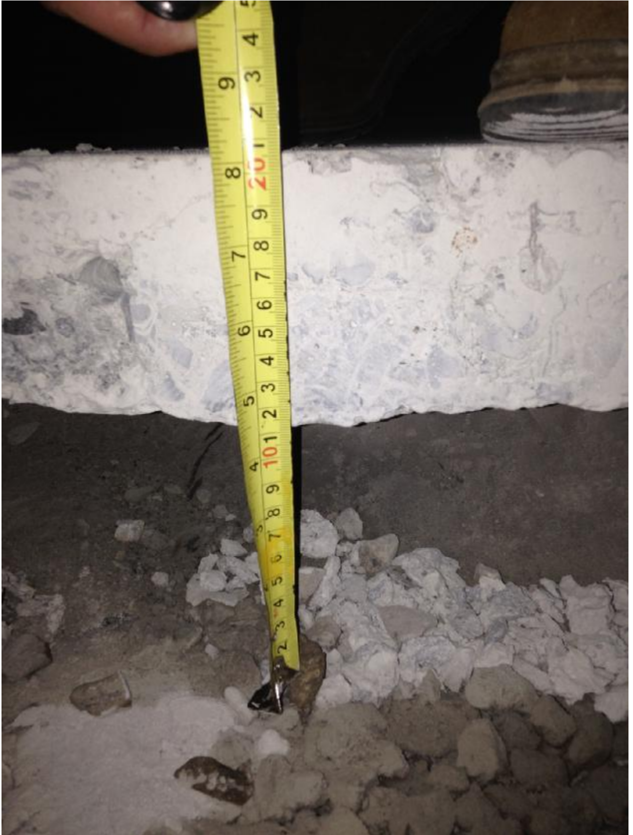
Photo 17 – Void under slab
