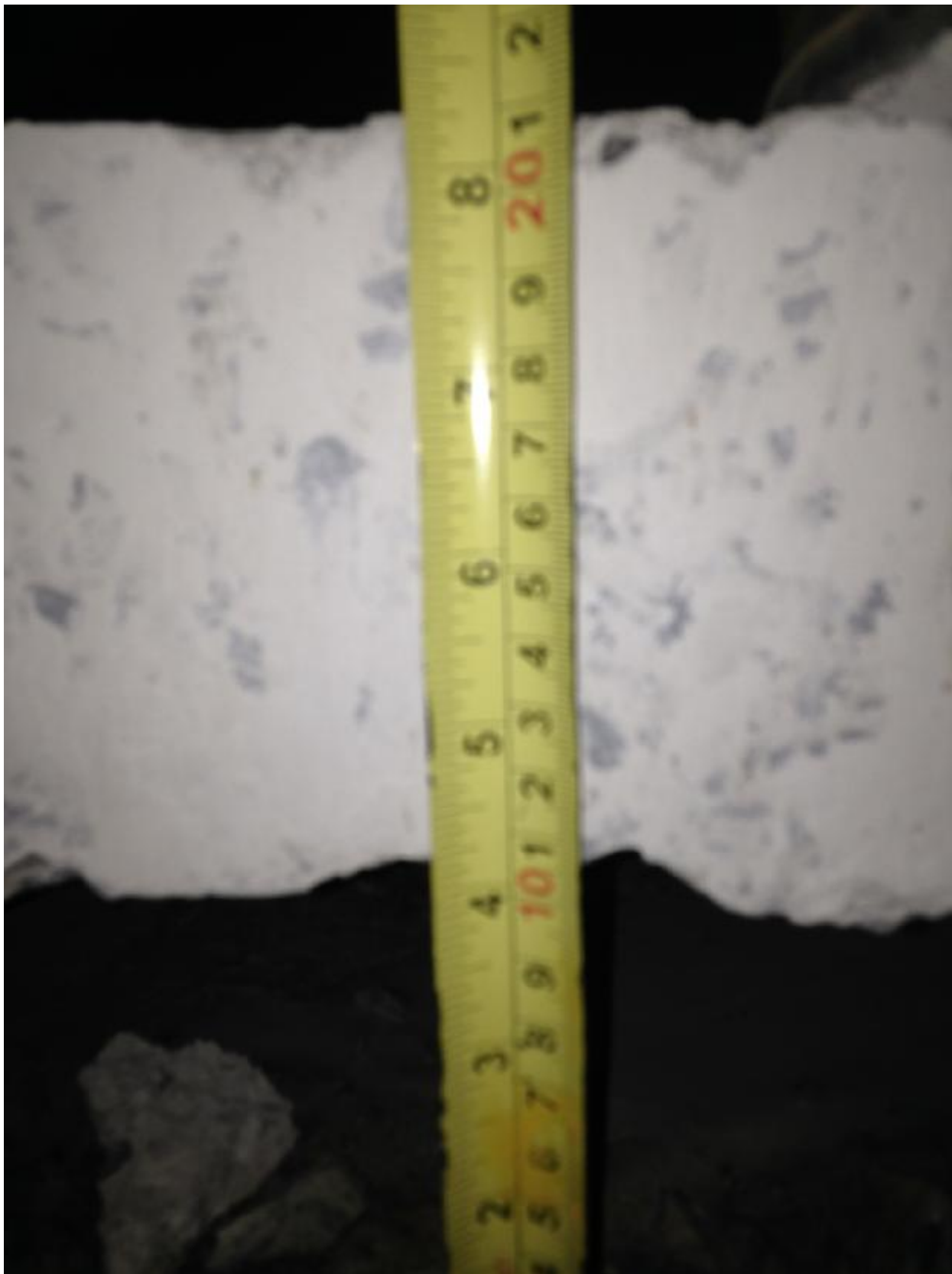
Photo 16 – Depth of void 100mm
