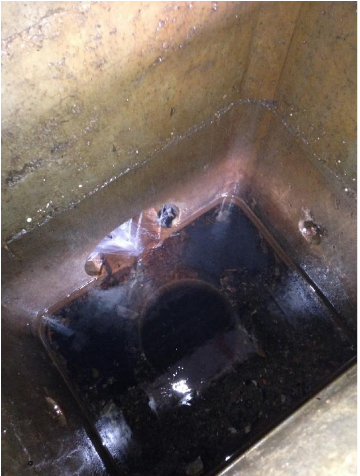
Photo 2 – Ground water entering around pipe penetration in the Ecosol Unit on basement drainage system located in loading dock
