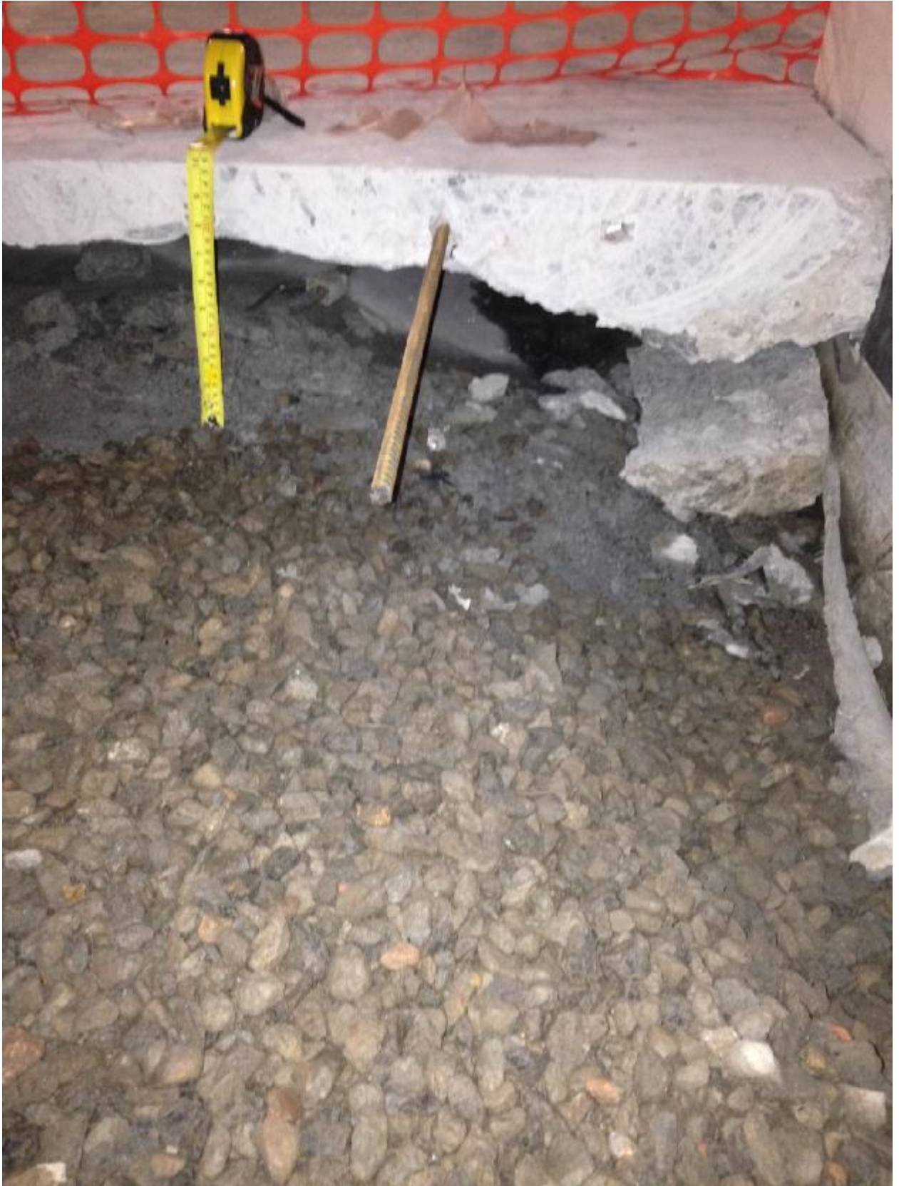
Photo 8 – Void under slab. Slab thickness only approximately 80mm thick
