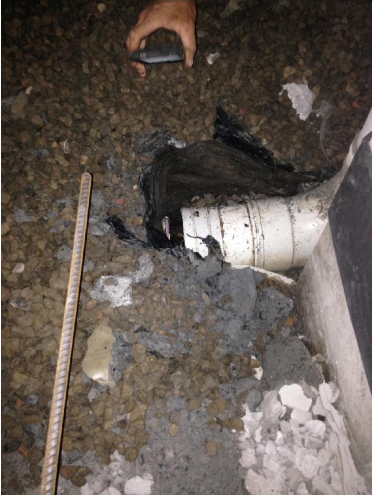
Photo 12 - Broken roofwater pipe
