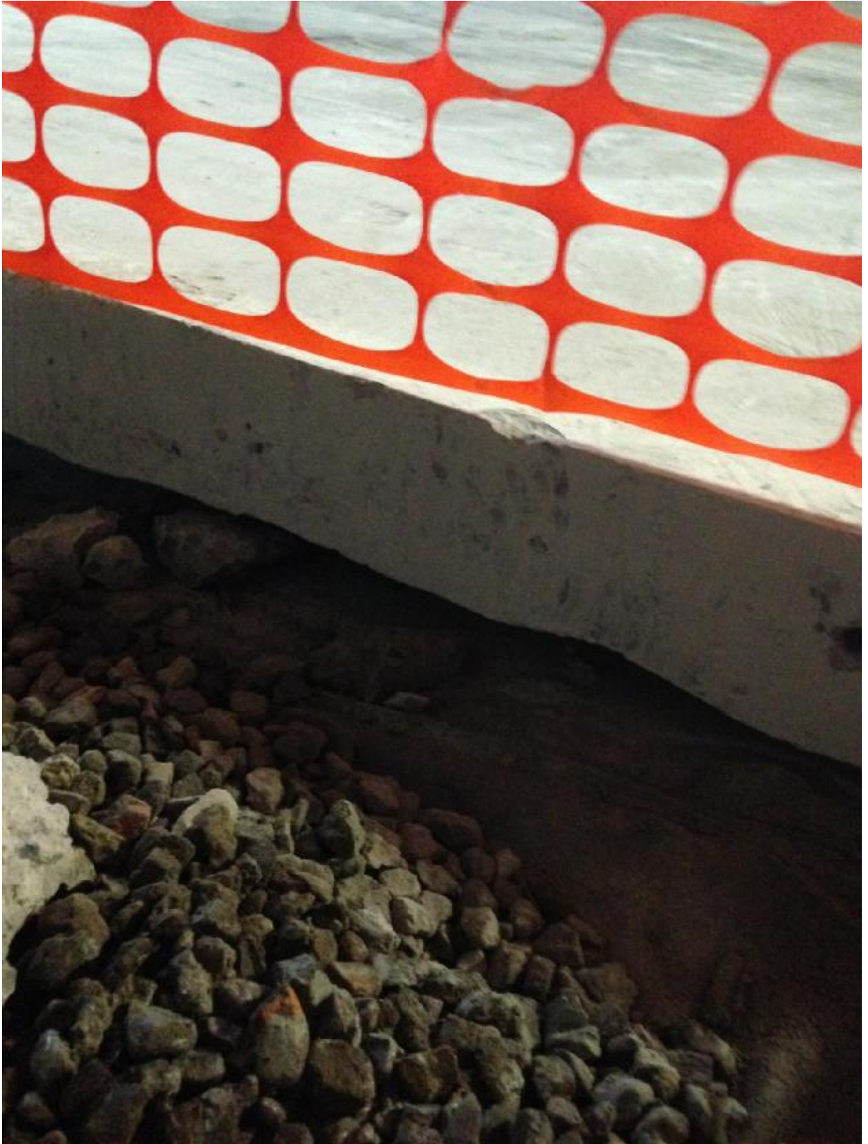
Photo 15 – Void under slab
