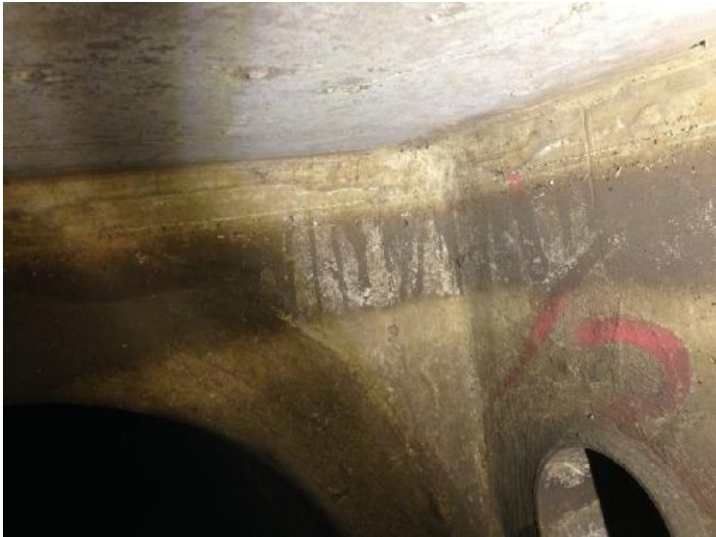
Photo 1 - Manhole on sealed roof water system. Aspro Slab still connected and sealed to main chamber
