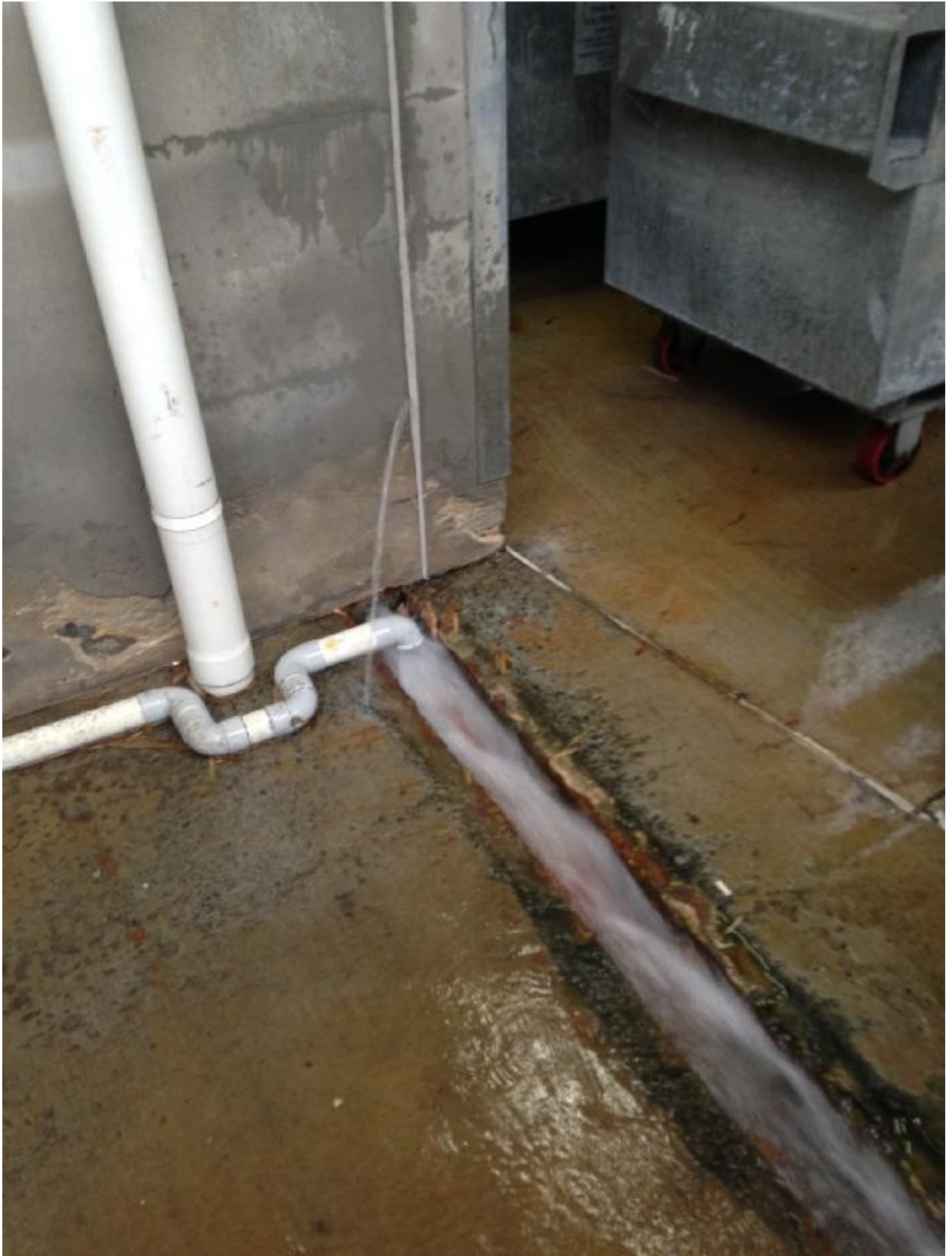
Photo 3 – Discharge to loading dock area from under basement slab
