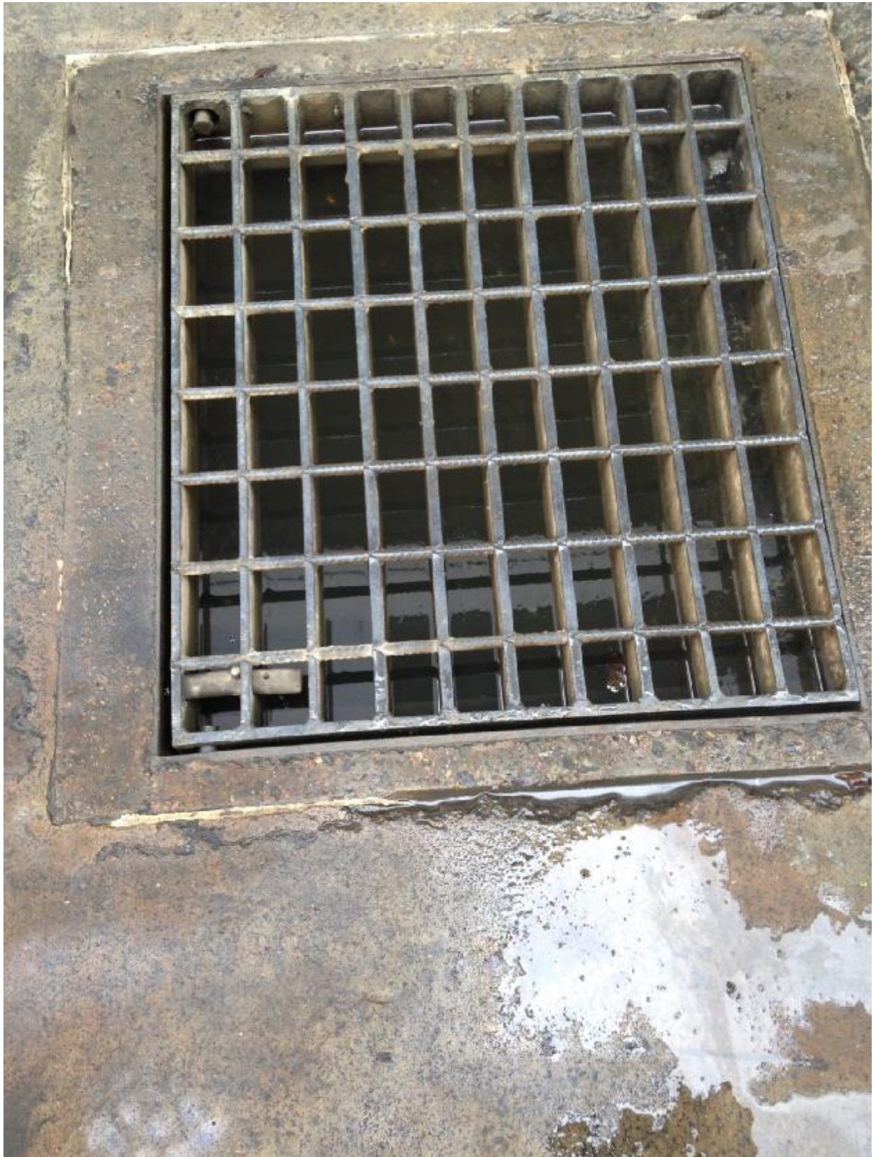
Photo 3 – Pit on basement drainage line located upstream of pumps in loading dock. Full of water due to non-operation of pumps
