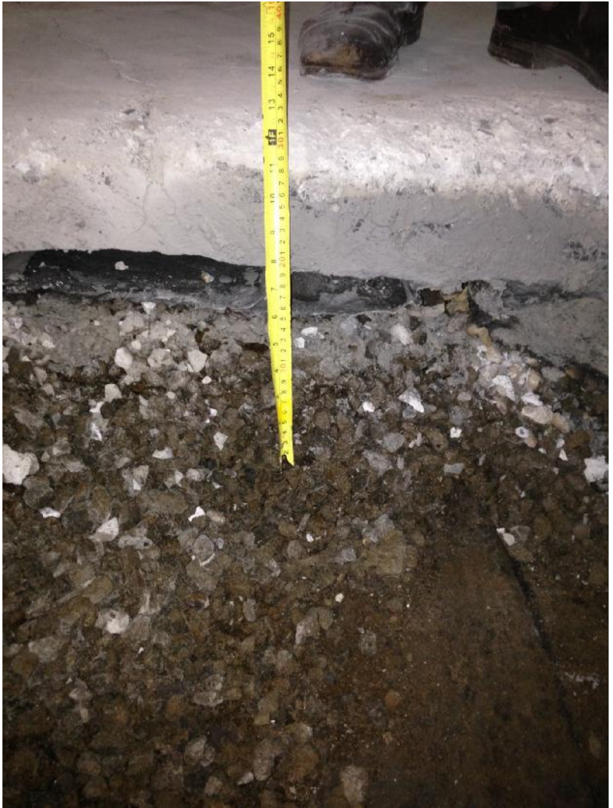
Photo 9 – Void under slab approximately 200mm deep
