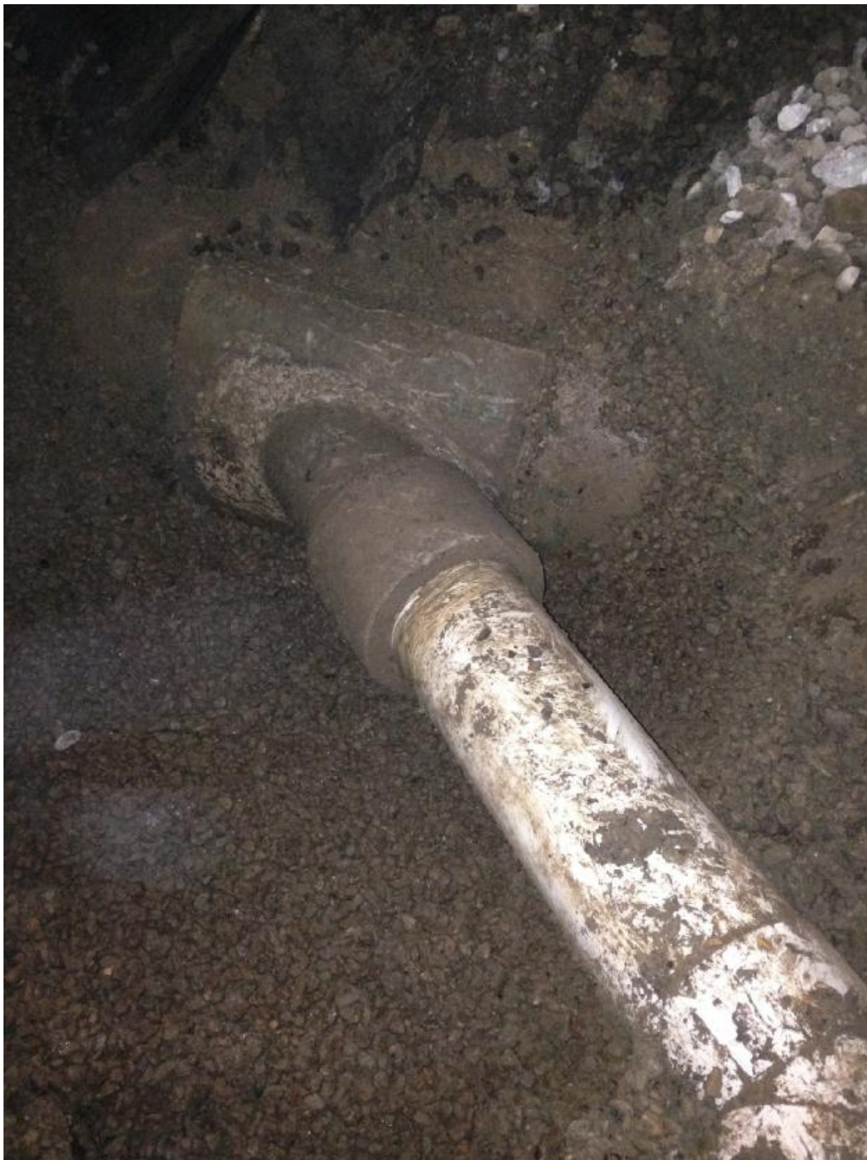
Photo 20 – 150mm roofwater saddle joint to 525mm diameter pipe
