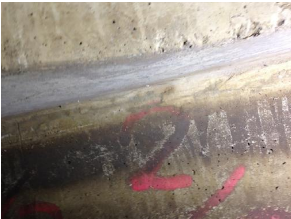
Photo 2 – Manhole on sealed roof water system. Aspro Slab still connected and sealed to main chamber
