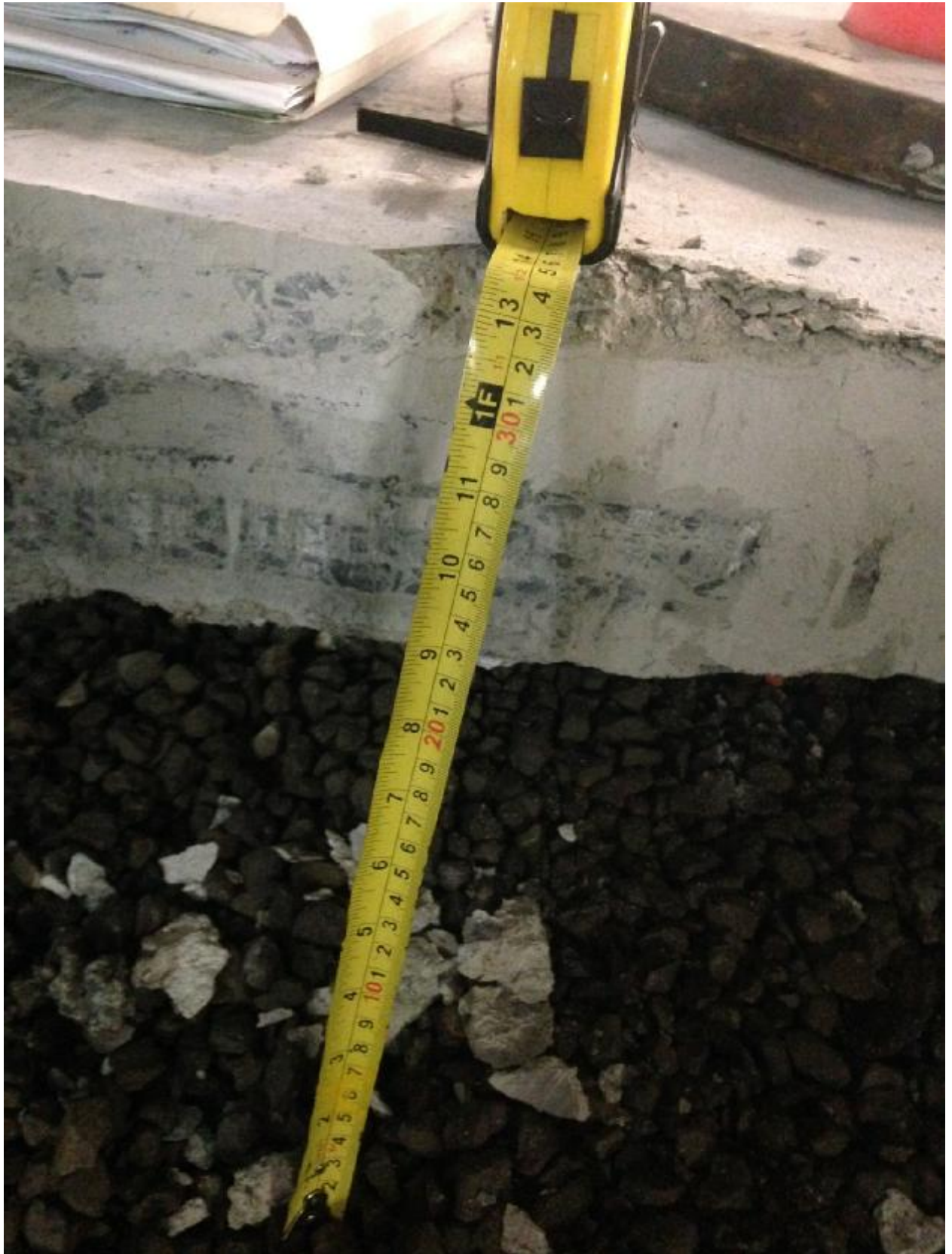
Photo 2 – Void under slab
