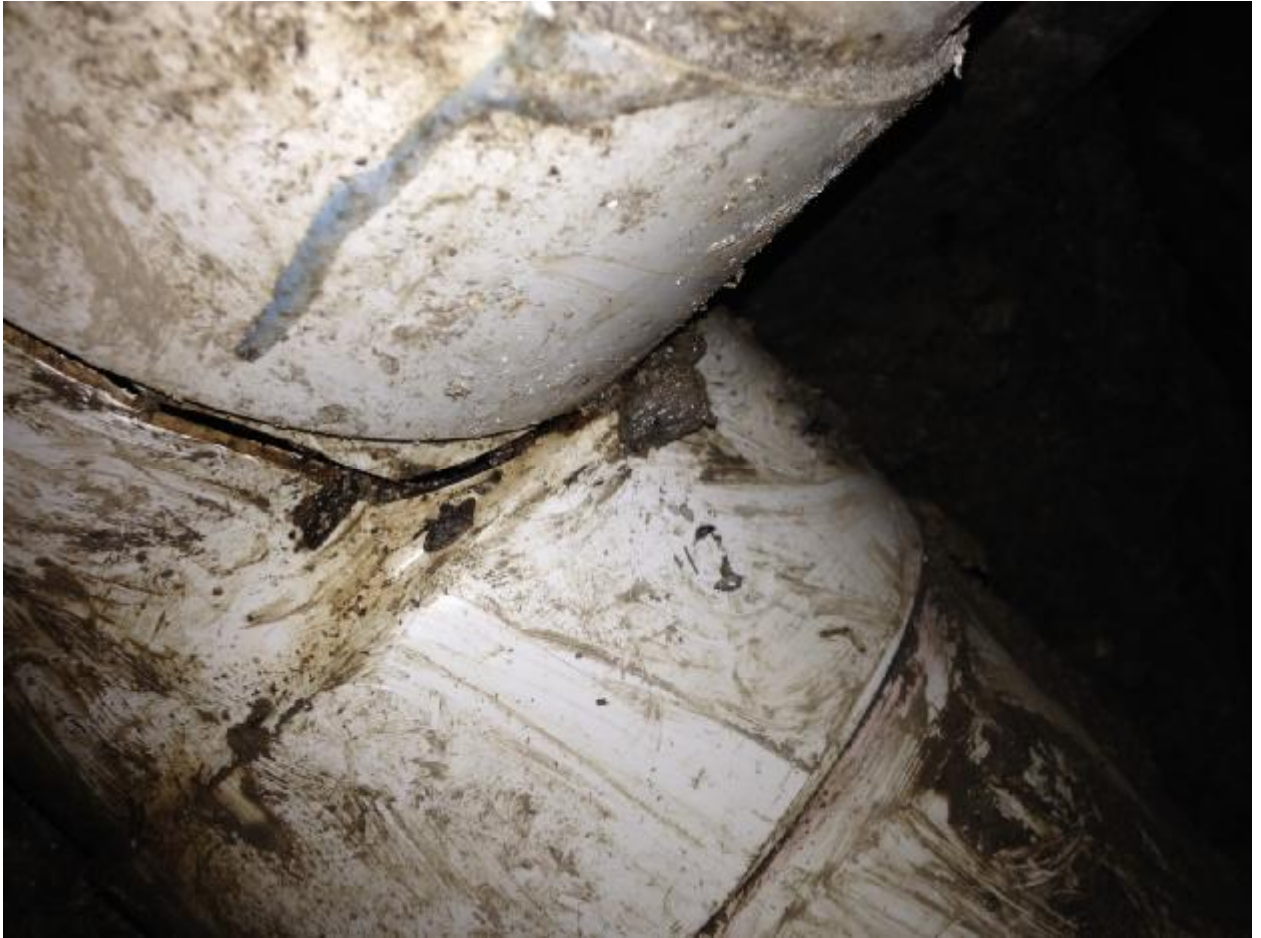
Photo 19 – Close up of broken roofwater pipe
