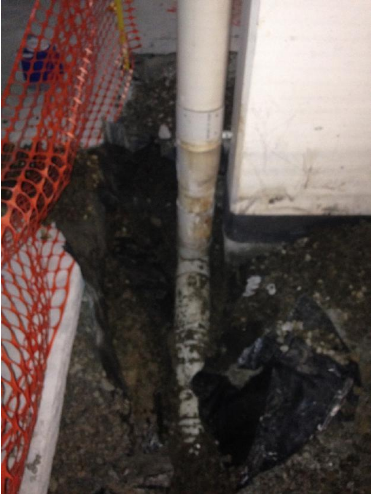
Photo 18 – Cracked roofwater pipe wide shot
