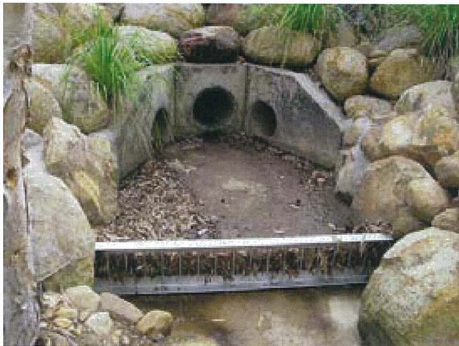
Figure 3-6 Example of a Trash Rack
