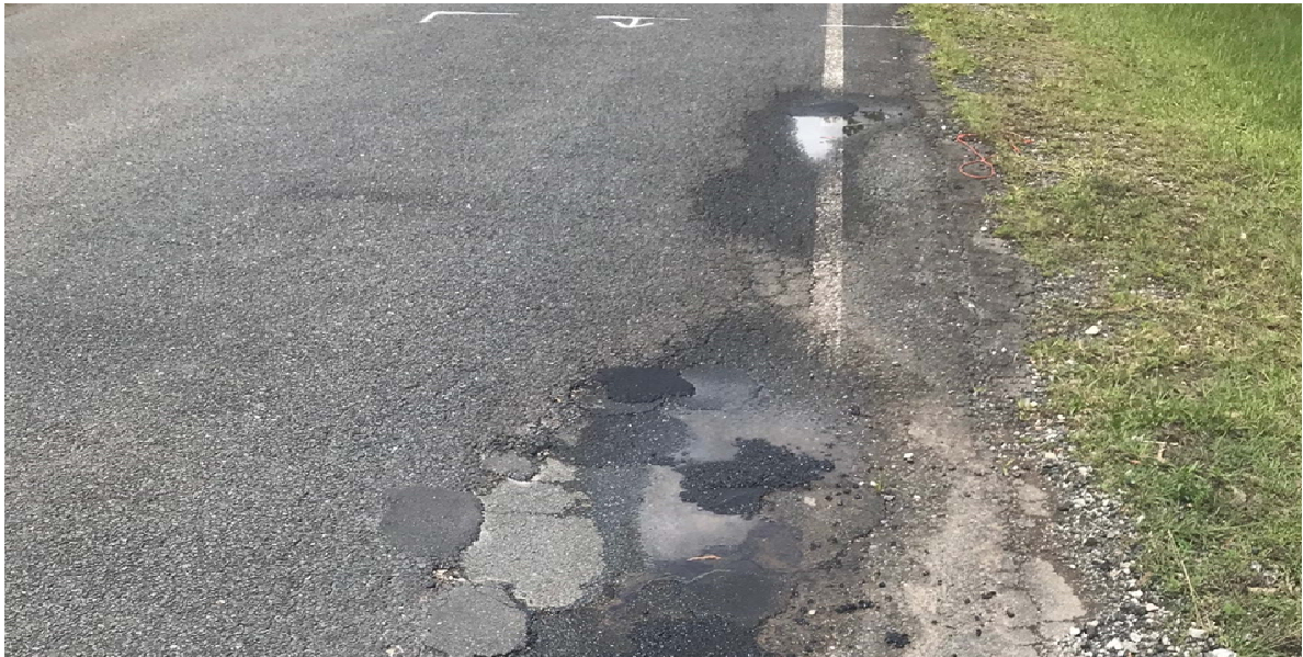
Figure 2-10 Intermittent pavement deterioration
