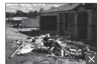
Poor litter and building waste storage
