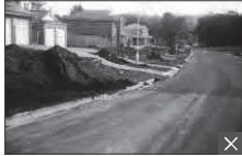
Stockpiles without protection
