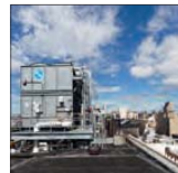
Unconcealed building services and mechanical equipment visible on tower rooftops
