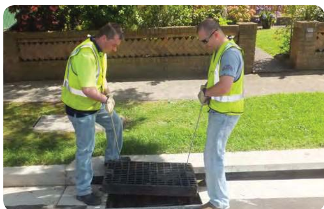
Photo 9 Lift grate above the support frame
