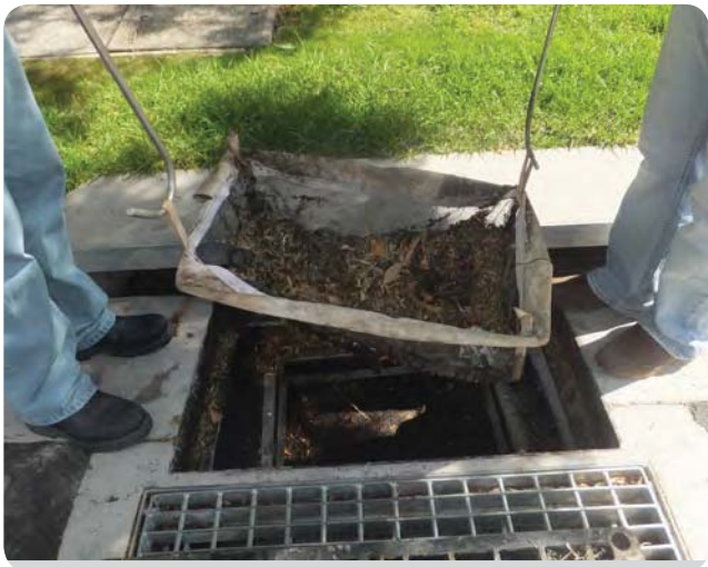
Photo 14 Lift the bag from the stormwater pit
