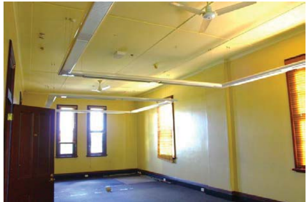
Figure 19 – Typical First Floor Office Fitout with Air Conditioning Unit
