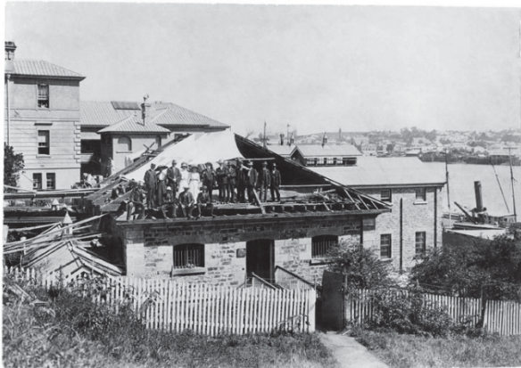
Figure 11 – Construction of third level, c.1912 also showing entrance to second storey via Miller Park
