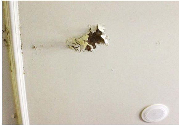
Figure 29 – Exposed fibrous plaster, Second Floor
