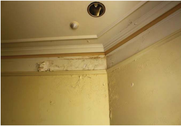
Figure 28 – Typical water damage, Second Floor
