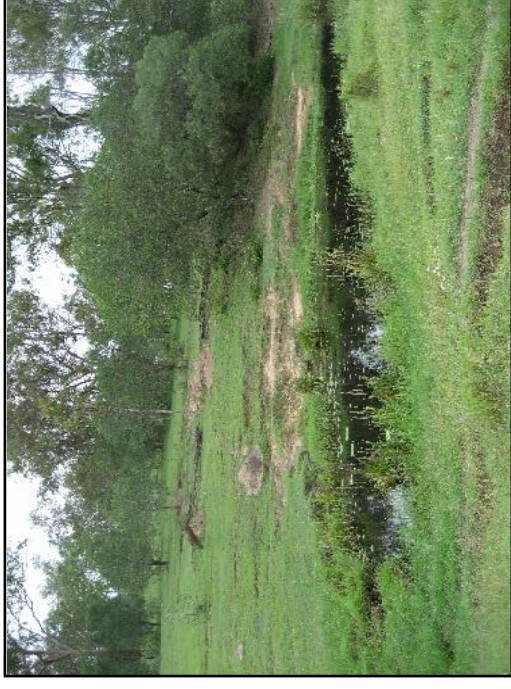
Plate 9 - Ponded water in drainage feature with minor slips and slumping along banks.
