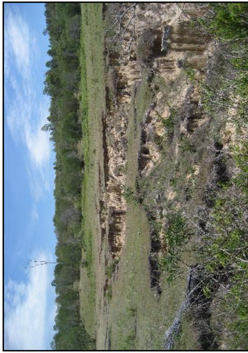
Plate 4 - Highly eroded drainage feature with no vegetation evident.
