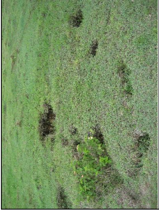
Plate 11 - Sink holes within flat drainage feature.
