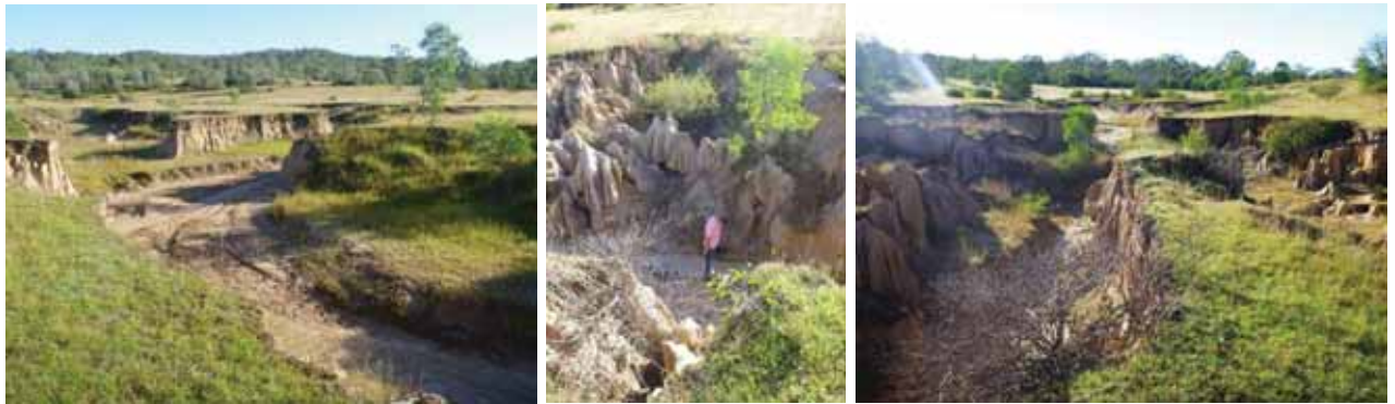
Examples of 3-5 m deep eroded drainage paths in the upper to mid catchments
