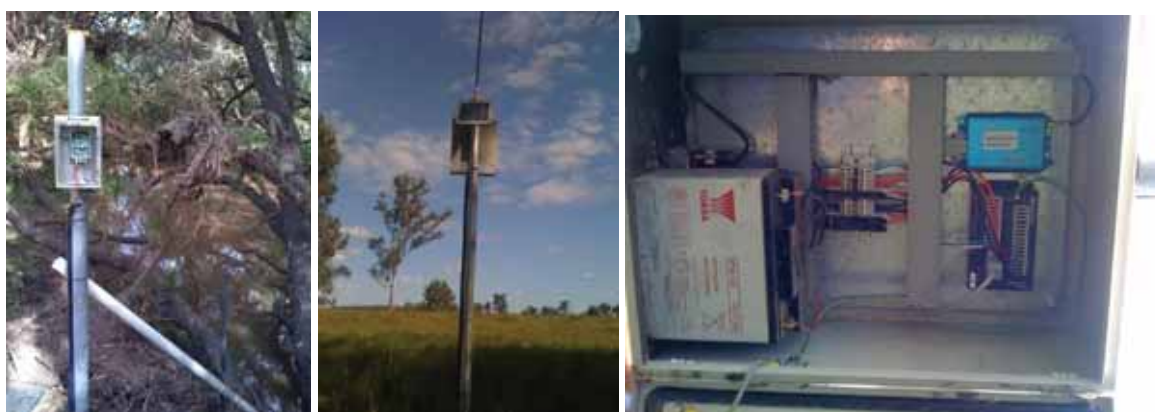
Figure C-1 Photos of Telemetered Water Quality Monitoring Infrastructure
