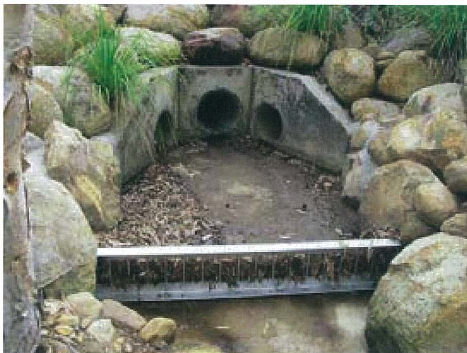
Figure 3-6 Example of a Trash Rack
