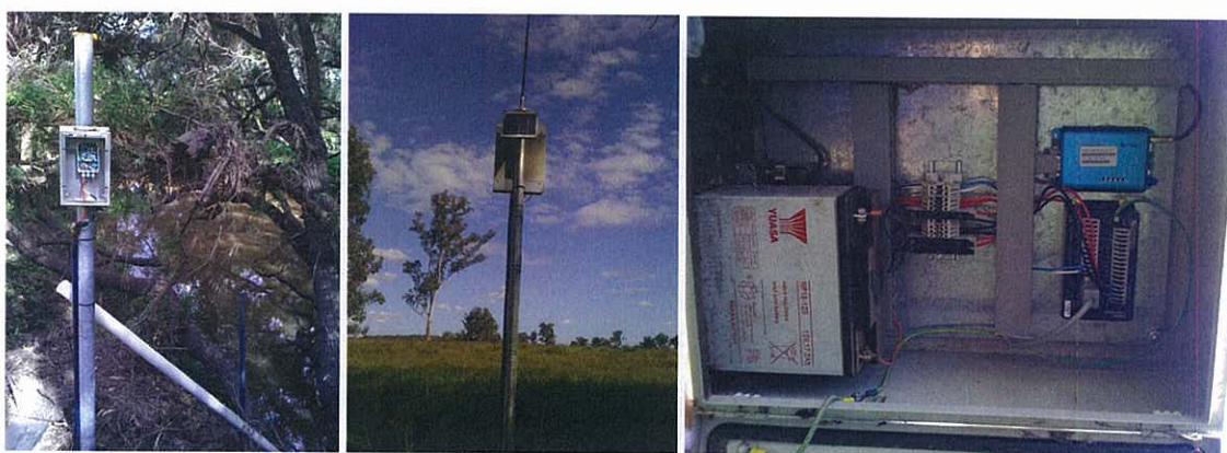
Figure I-1 Photos of Telemetered Water Quality Monitoring Infrastructure
